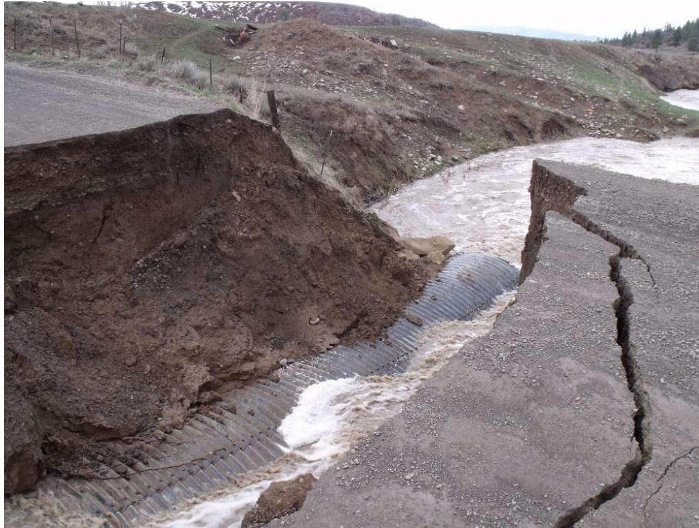
Figure 4 .14. April 17, 2010 Flood and Culvert Washout Along Stollsteimer Creek
